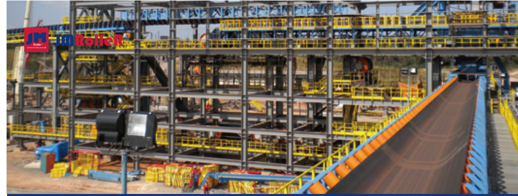
Belt Conveyor Machine
