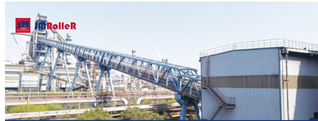
Belt Conveyor Machine
